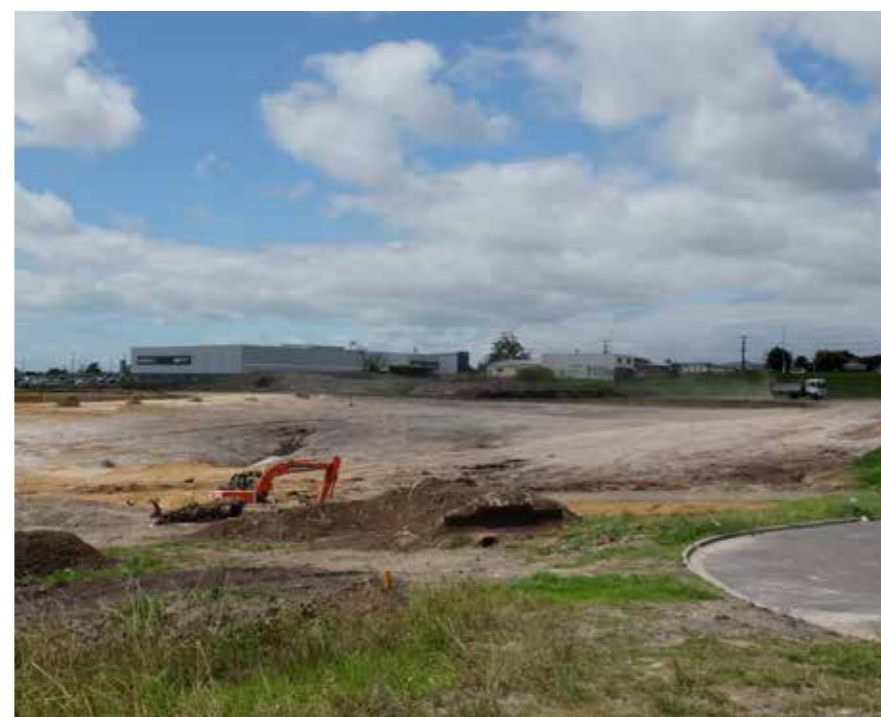
14. This photo was taken from MT15 with Sinton Road to the right. Development of the surrounding area is under construction.
